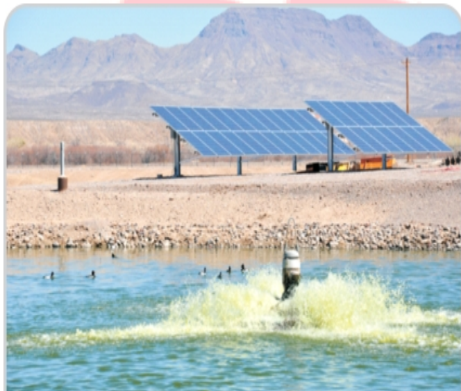
Solar pumps provide pond aeration for water treatment or for aquaculture
