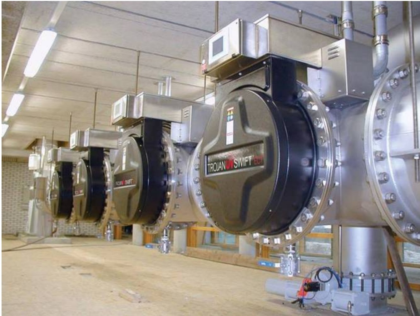
TrojanUVSwift™ ECT installation in Andijk (1 train of 3 trains)
