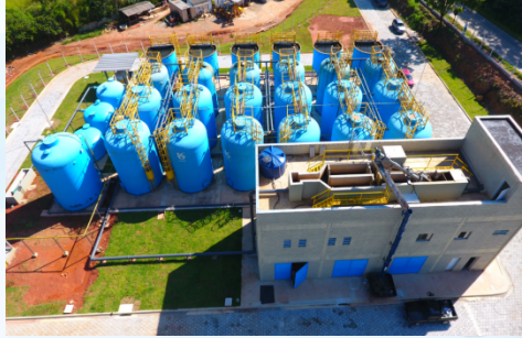
ETE Alumínio - Q=36,0 l/s
