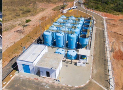
ETE Águas de São Pedro - Q=36,0 l/s
