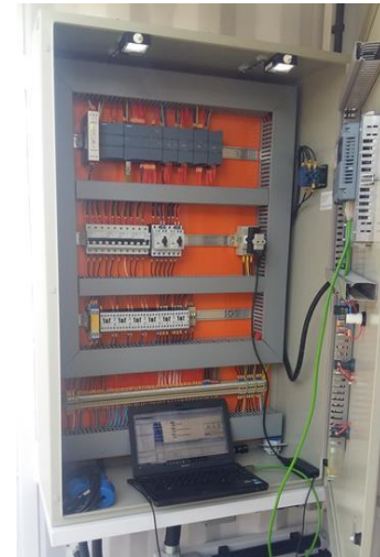
Painel de controle
