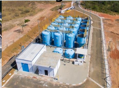
ETE Águas de São Pedro - Q=36,0 l/s
