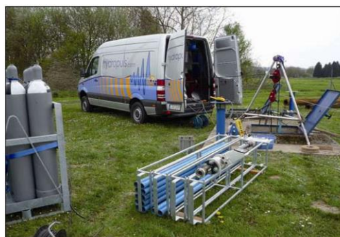
Well and borehole intensification with hydropuls®
